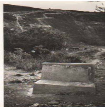
The pipe from the filter/intake box is mortared onto the rock until it reaches the tap stand.
