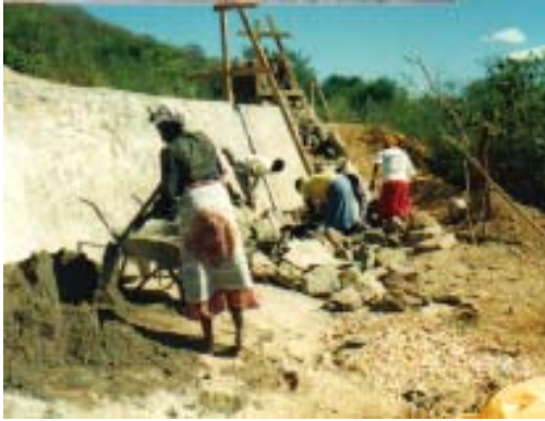
The first stage of a masonry wall being extended by a second stage.
